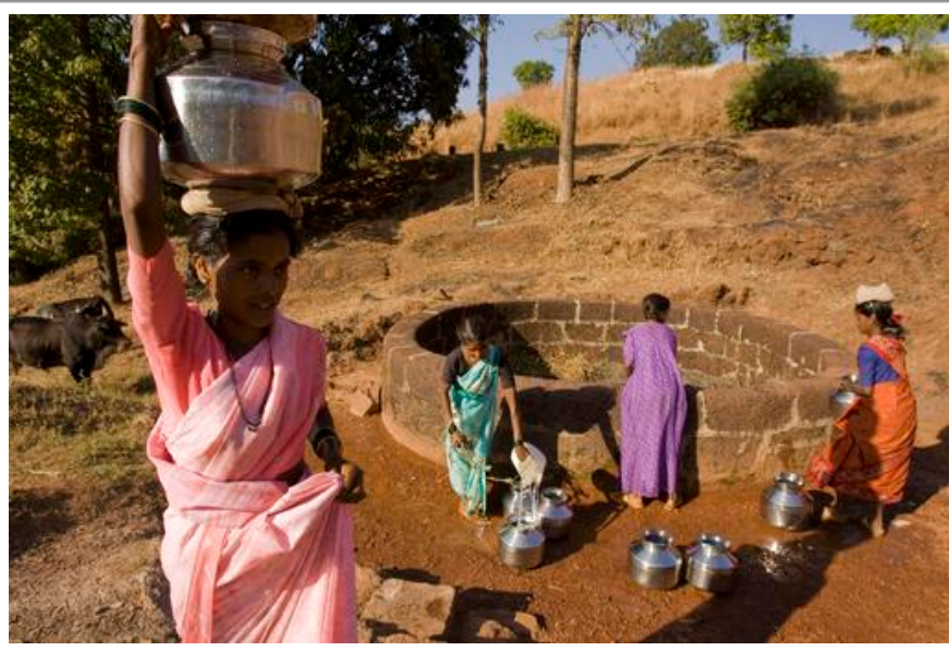
People from Mandatane, India, work together with Rotarians to build a retaining wall. The rain water harvesting technique keeps the wells from going dry so they can yield all year. The Rotary club of Bombay Metro and Rotary Club of Palo Alto, California used an RI Matching Grant to facilitate the project.
